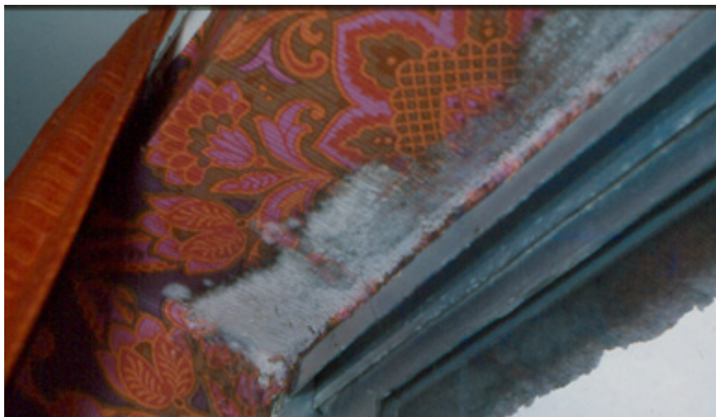
Figure 5 - Rain penetration around a poorly installed window frame
