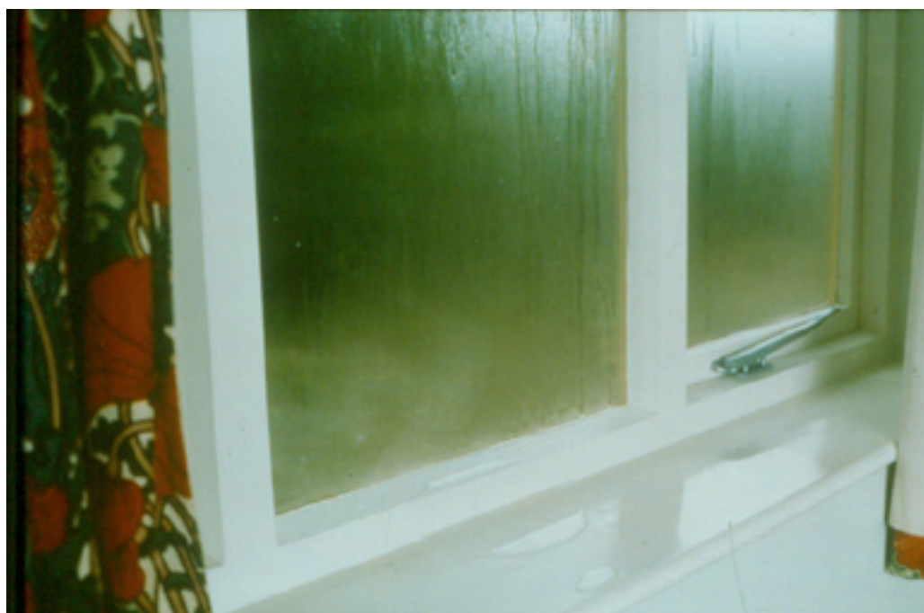
Figure 3 - Severe condensation on a window running onto the sill
