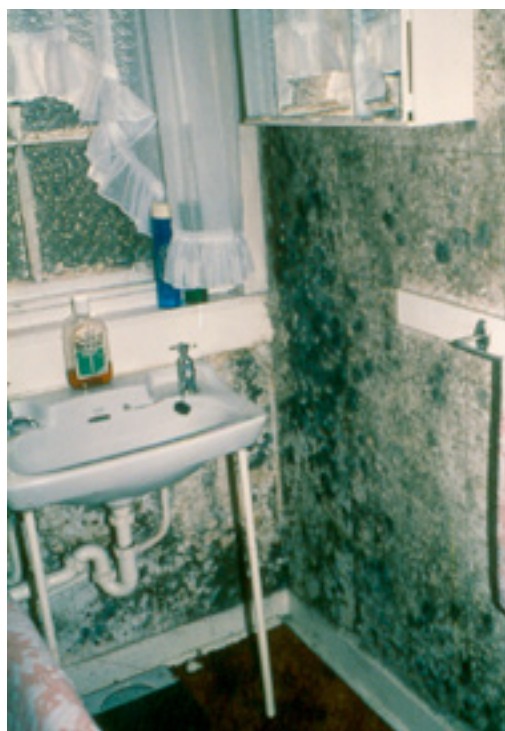
Figure 4 - Severe surface mould growth in a bathroom
